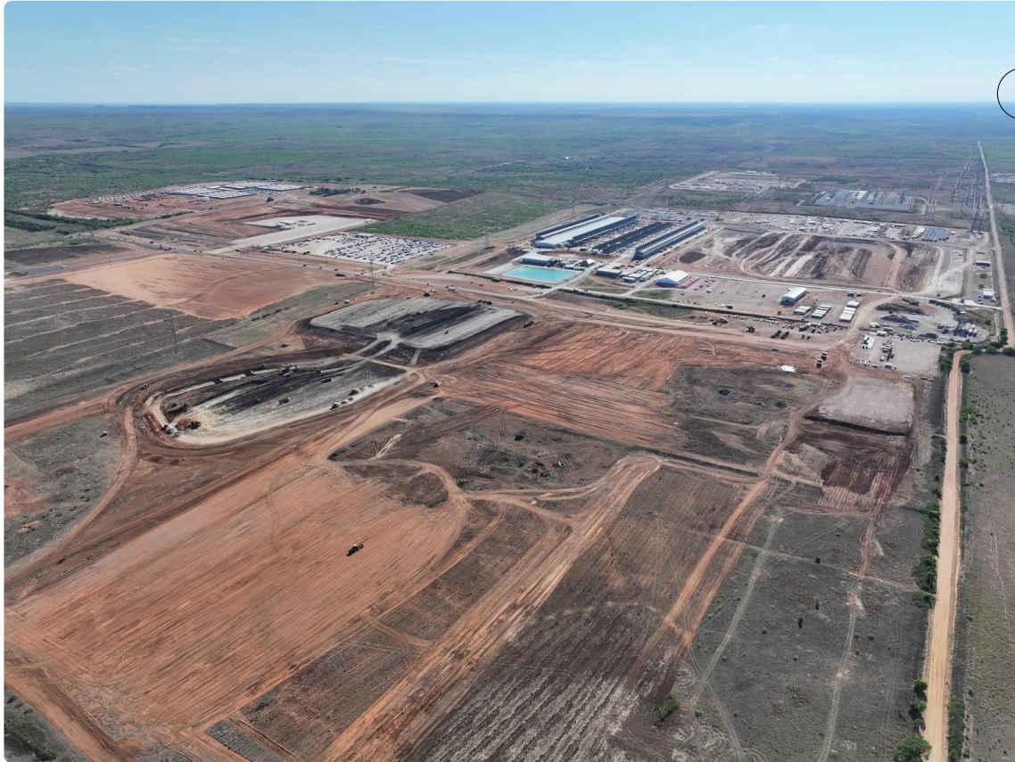
Galaxy's Helios Data Center campus, April 2026.
