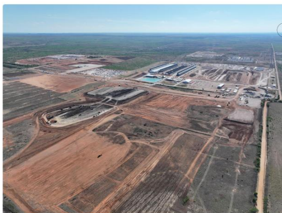
Galaxy's Helios Data Center campus, April 2026.
